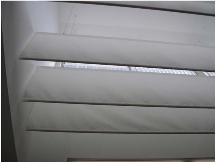
Figure 7. A view looking up into the roof monitors at Smith Middle School. This view shows the diffusing baffles hanging from the ceiling of the monitor.
