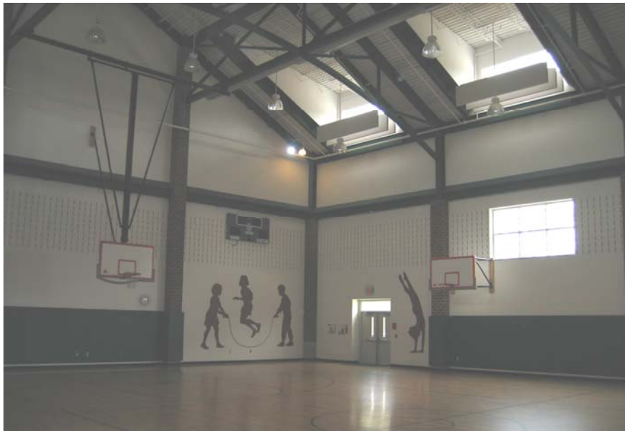
Figure 14. Baffles located on north facing windows high above the gymnasium floor do not serve a useful purpose and block light from entering the building at Rashkis.
