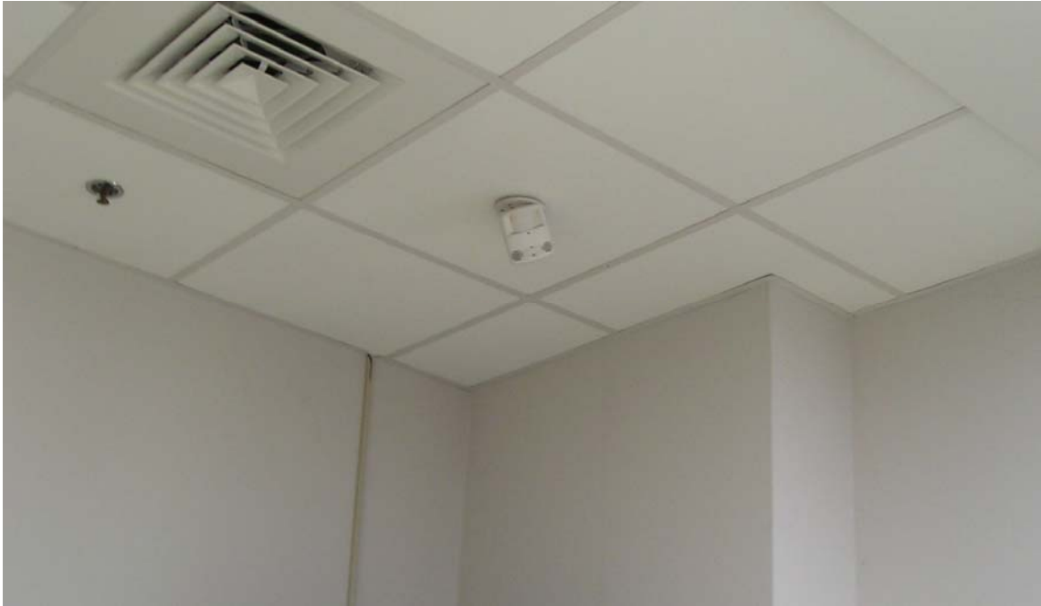
Figure 11. Occupancy sensors are located in most classrooms at Rashkis Elementary
