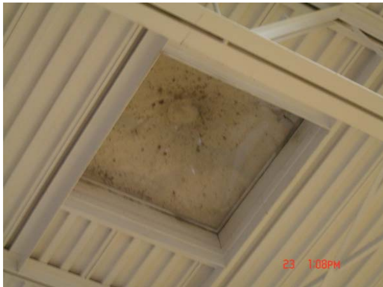
Figure 16. Skylights were covered when the roof was replaced on the gymnasium at Four Oaks Elementary School.
