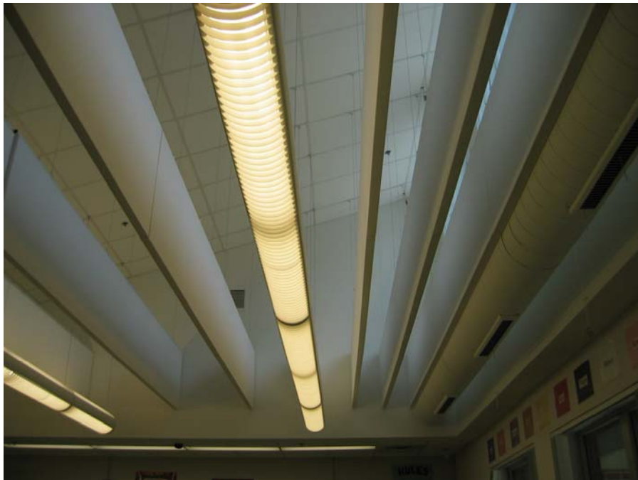
Figure 10. On south facing clerestories, cloth covered baffles diffuse and reflect the light down into the classroom. Note the placement of the fluorescent tubes between, parallel, and below the baffles.
