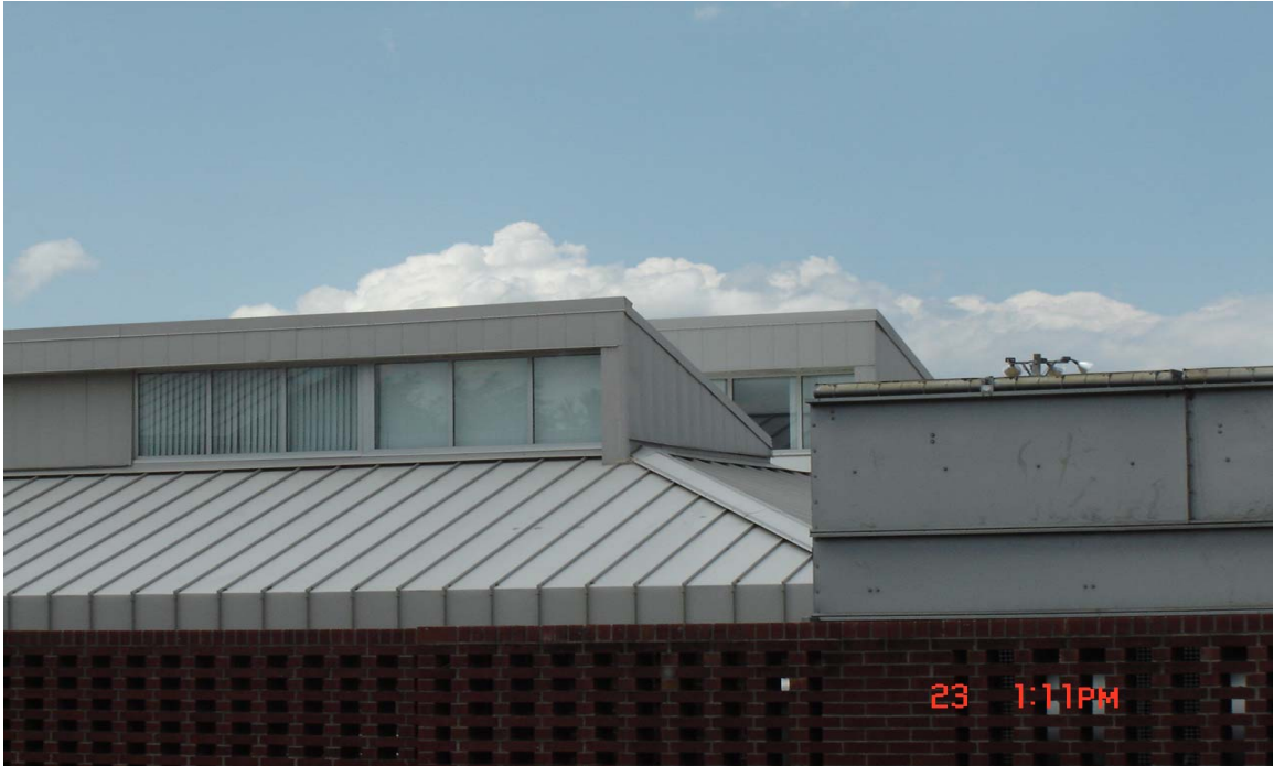
Figure 1. Front of clerestories at Four Oaks Elementary School. Note the lack of consistency regarding the position of the blinds.
